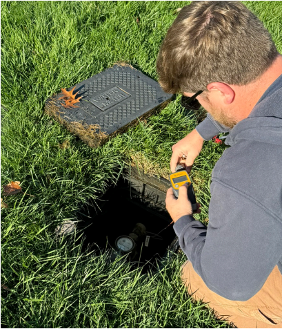
An HCWD2 employee is inspecting a water meter box.
